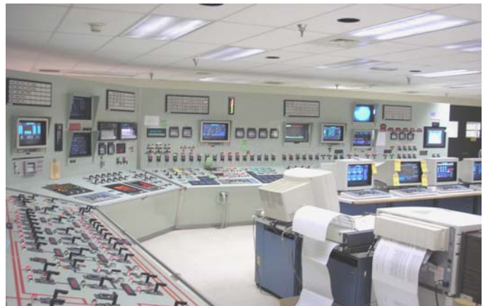
J. K. Spruce Control Room The Brain of the Power Plant
